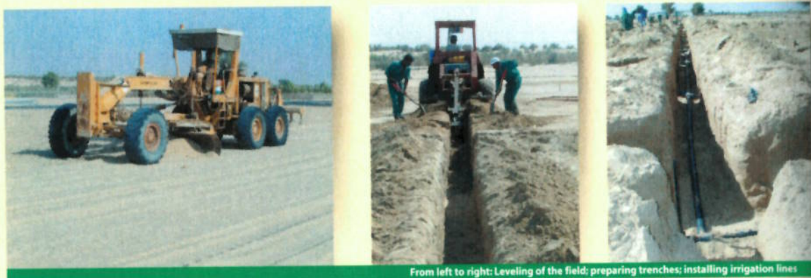
From left to right: Leveling of the field; preparing trenches; installing irrigation lines
